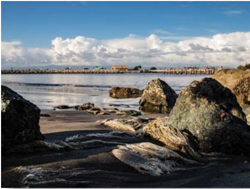
16-Plastic sand bags deteriorating into Moss Landing Harbor and our Marine Sanctuary.JPG
