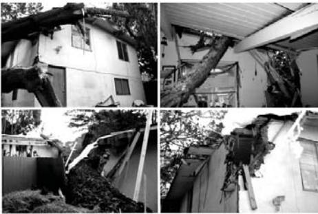
08-Fallen Tree Damages House during Storm.jpg
